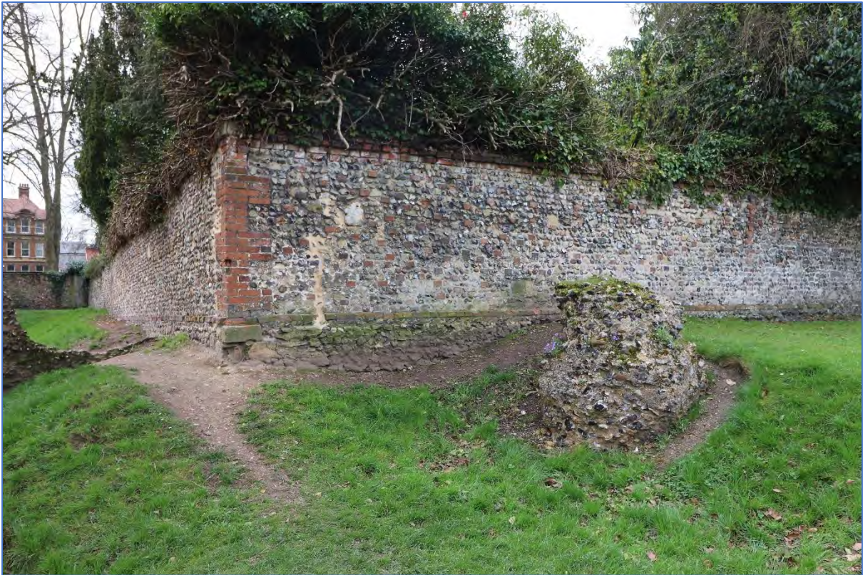
Figure 107: The eroding foundations of the north-eastern corner of the Deanery's garden wall, which was clearly constructed on top of the post-Dissolution rubble layer.
