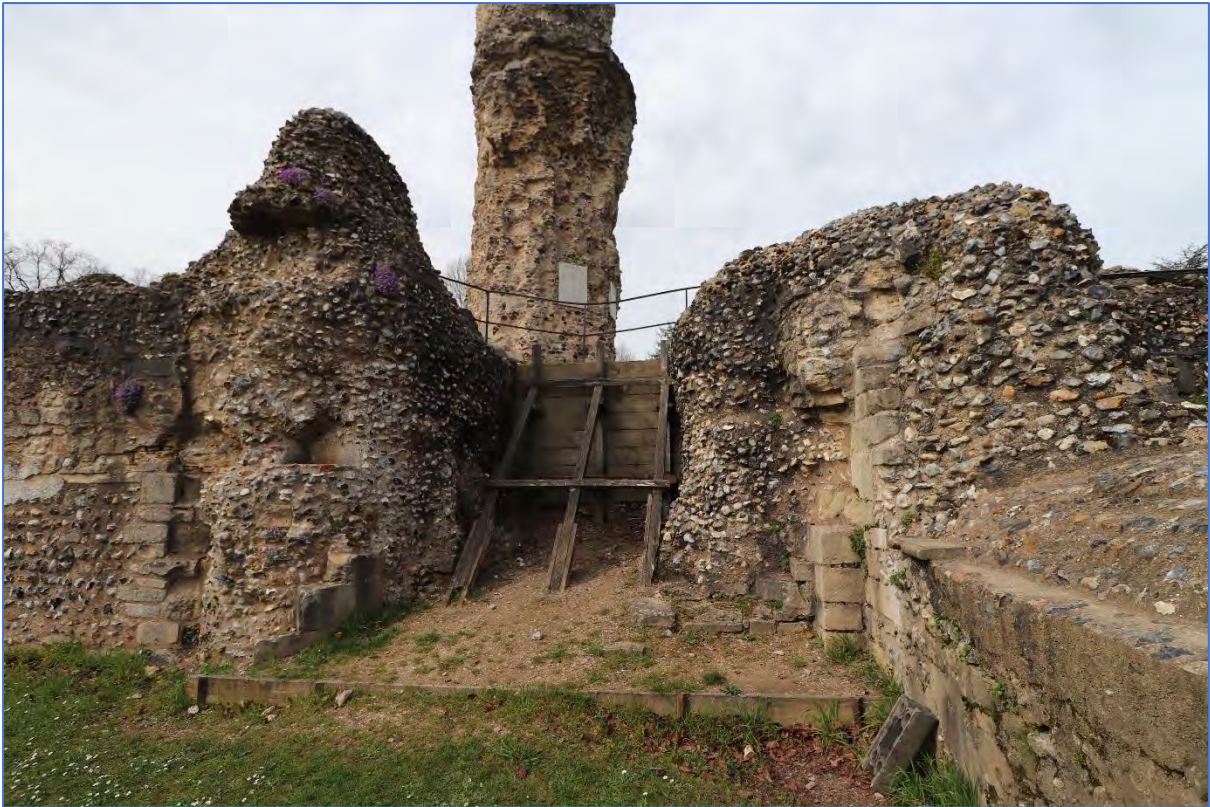
Figure 98: View of the position of the staircase leading from the north transept to the crypt, looking west, showing the wooden shuttering now used to support the backfilled passage..
